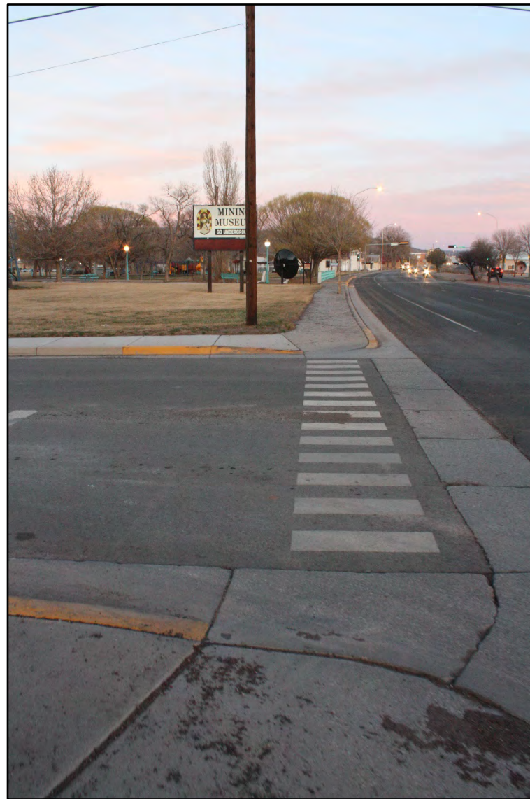
Figure 12. Non-ADA Accessible Sidewalk
